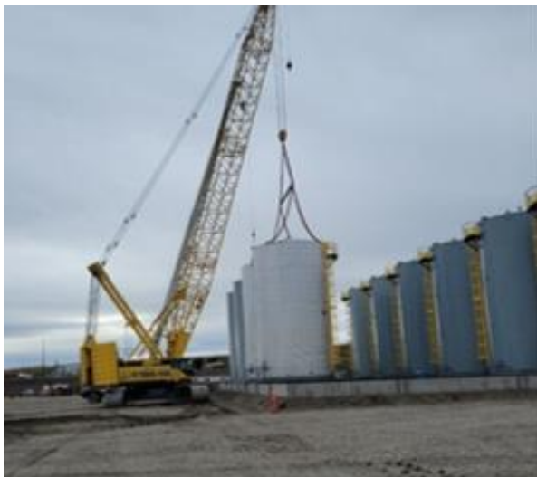
Tank Farm Installed
