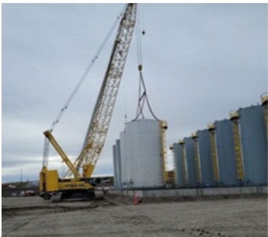
Tank Farm Installed
